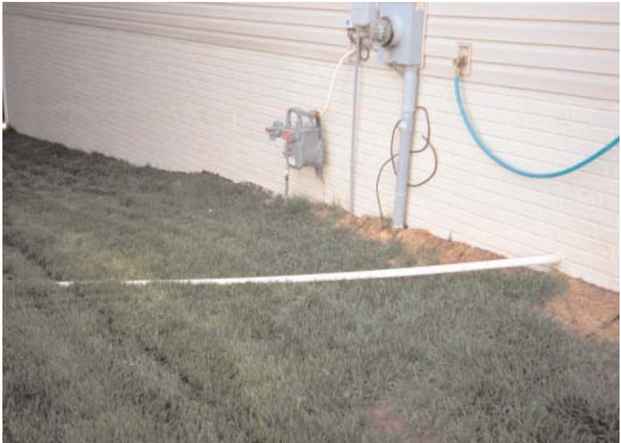
1-23 Exterior portion of sump pump discharge
