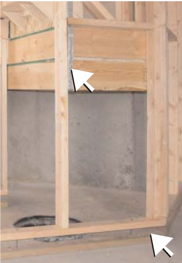
1-14a Floating wall hung from the floor above (note support strap and gap at bottom)
