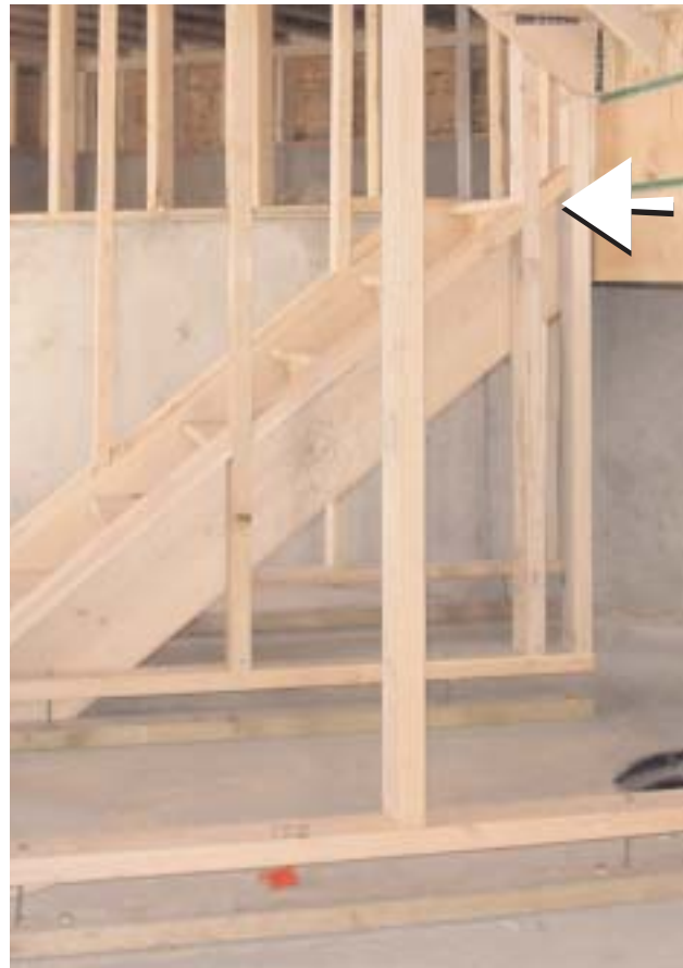
1-14b Hinging at the landing above (arrow) allows the staircase to adjust if the basement floor rises
