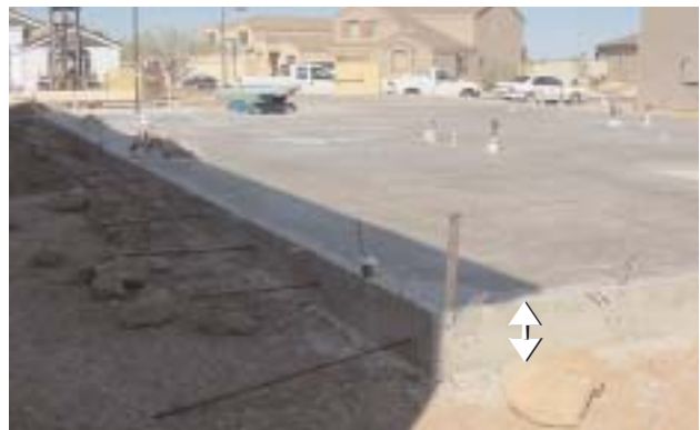
1-10 The perimeter may be twice as thick as the rest of the slab
